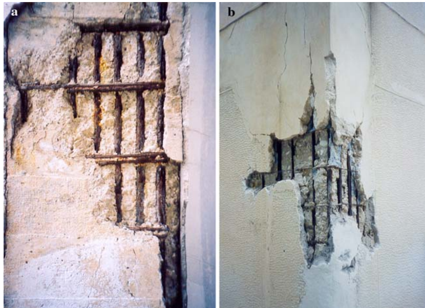
Fig. 3 Photos of deteriorated concrete structures due to reinforcement corrosion (a) Ladopoulos papermill, Patras, Greece (73 years old) (b) General Hospital, Lixouri, Greece (51 years old)
